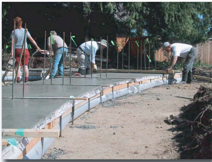
Terra Firma Builders (Salt Spring Island, BC) reduce forming costs and eliminate rising damp.
