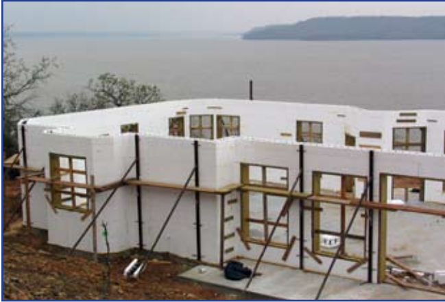
Minimal Outer Bracing
