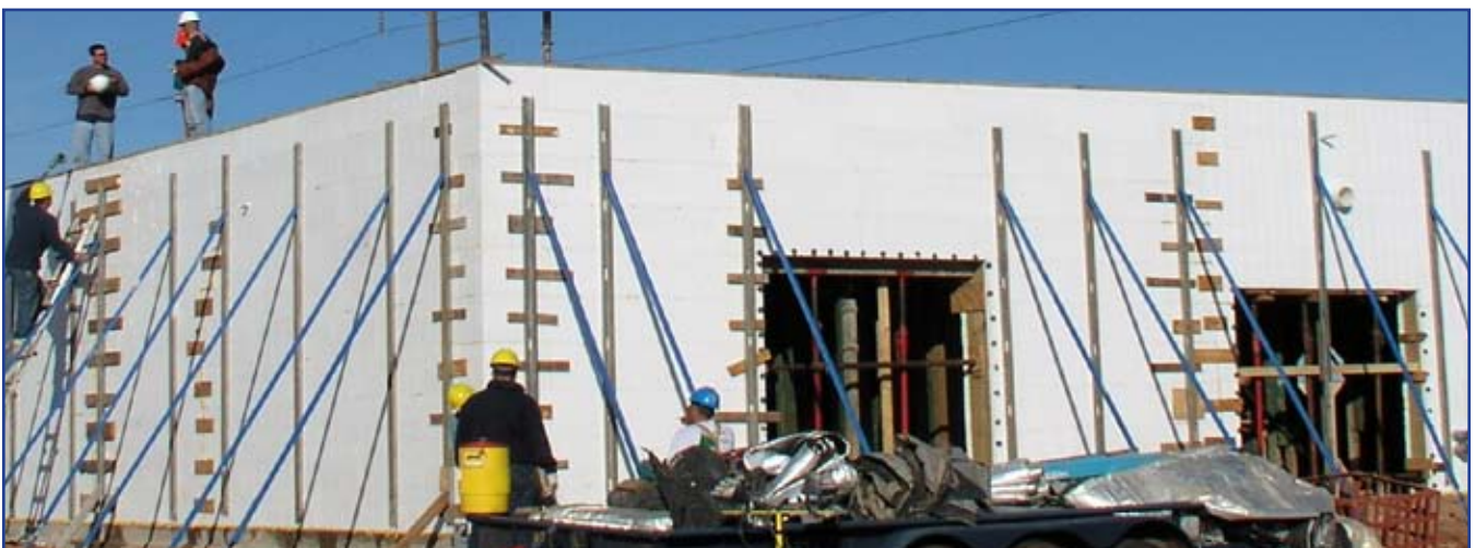
Ample Outer Bracing with "Scabs" on Non-Factory or Irregular Cut Joints (No Walk Boards)
